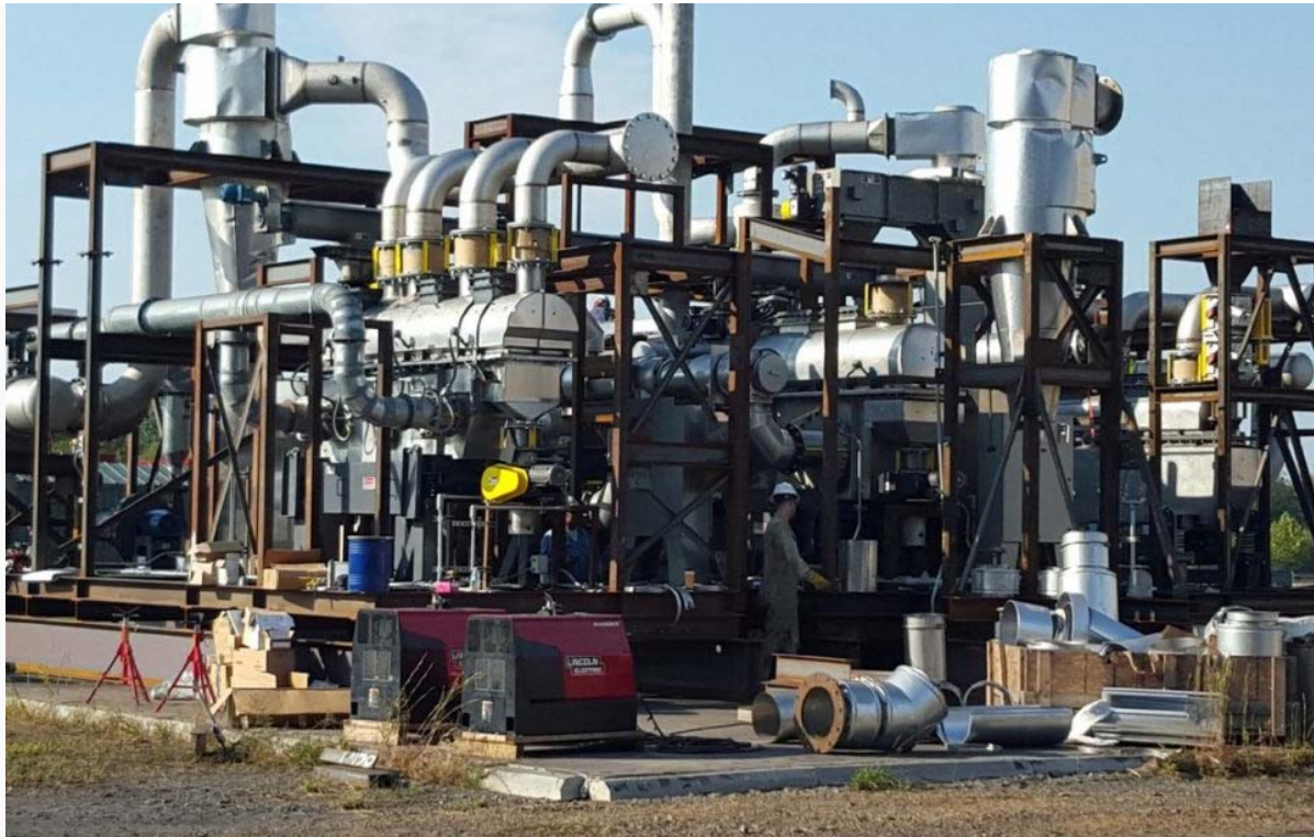
AES facility near Tulsa, Okla. before it was disassembled and relocated to Wyoming.
